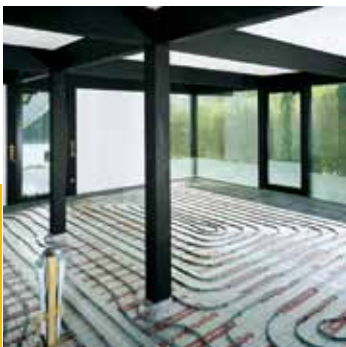
Underfloor heating living area
