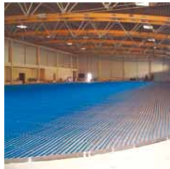
Chilled area, ice stadium
