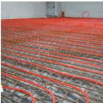
Industrial floor heating
