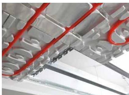
Installation and fitting of R883-1 panels and pipes along the preformed panel and head housings
