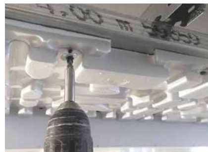
Installation and fitting of head panels on the metal support structure with 35 mm screws
