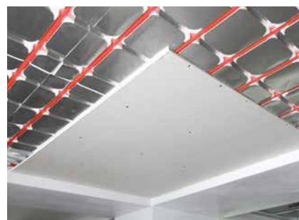
Installation and fitting of plasterboard sheets on the support structure after pressure test performed according to the rules in force
